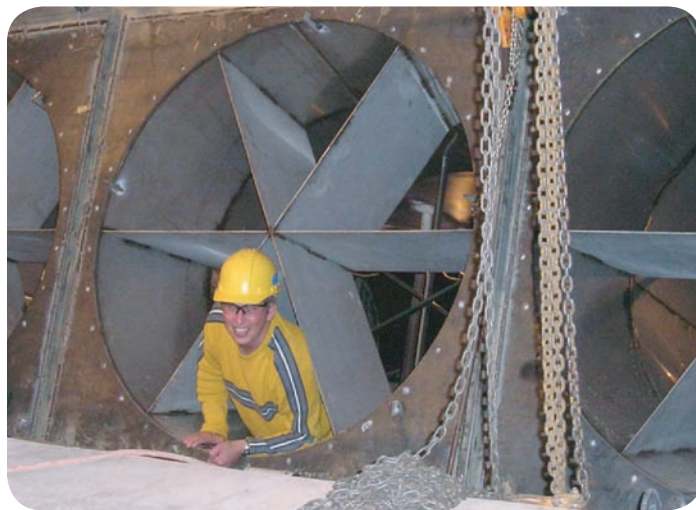
Installation of multiple High Beta® Elements within a rectangular duct, focusing on the straightening vanes
