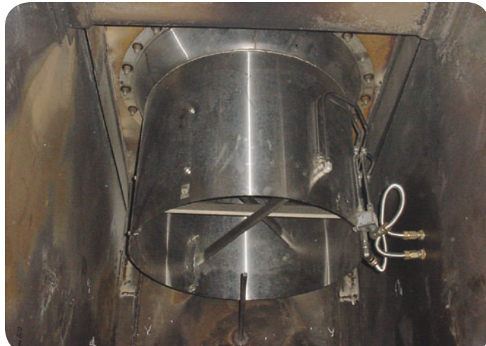
Installation of Eastern Instruments High Beta® in a rectangular duct
